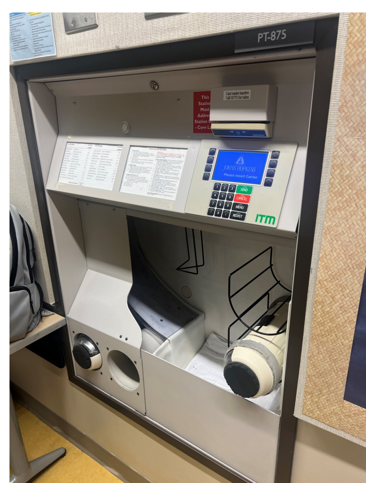
PICU Pneumatic Tube Station No. 845 with Two Capsules Visible
